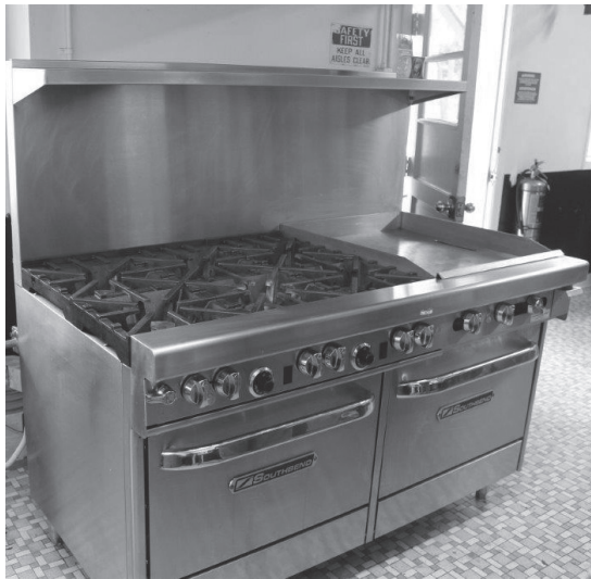
The new stove at the house.
